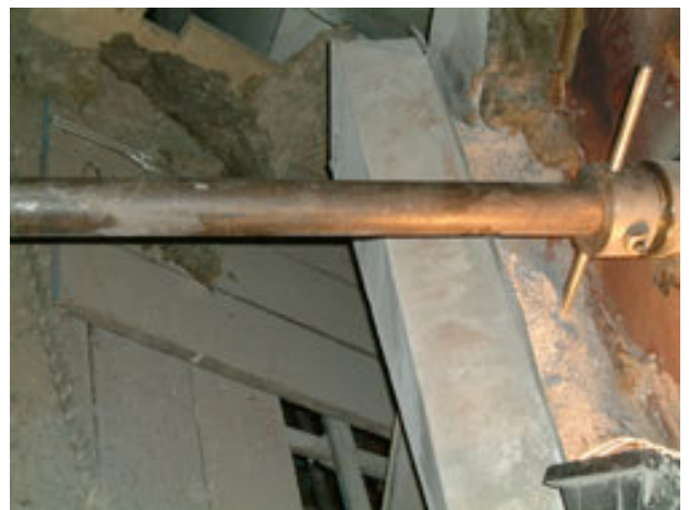
Cardox Tube inserted into Socket on 2nd floor of Economiser
