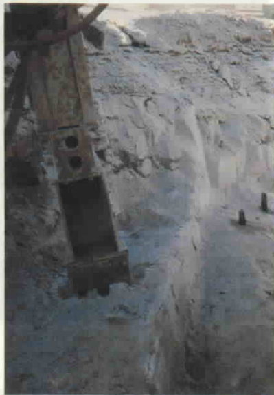
The Cardox sequence...holes are drilled in the homogenous granite and tubes inserted...
