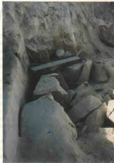
...and the excavator comes in handy for digging out the clean broken material.
